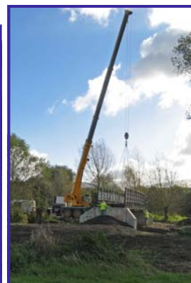
Construction of a bridge over the river, part of the Great Stour Way
